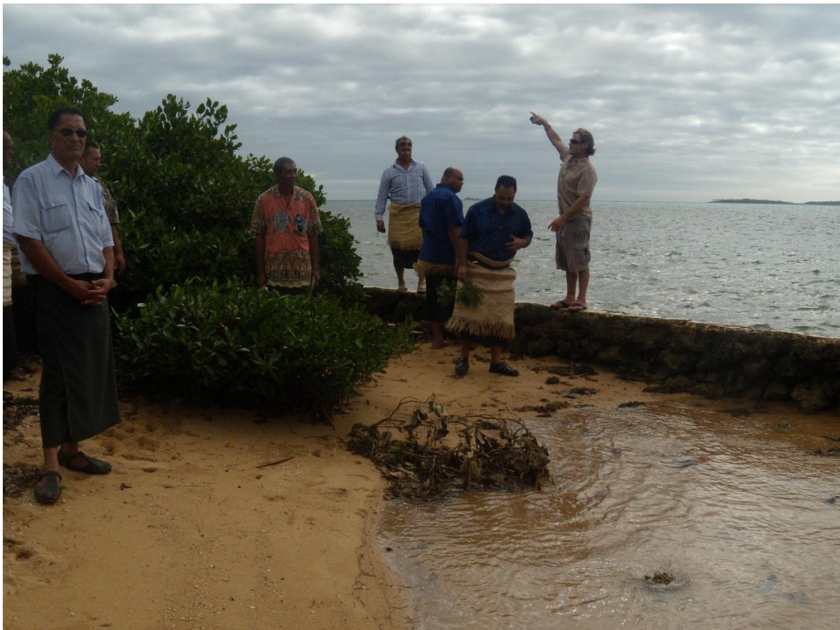
Workshop participants viewing a failed seawall and the colonisation of mangroves behind the failed seawall
