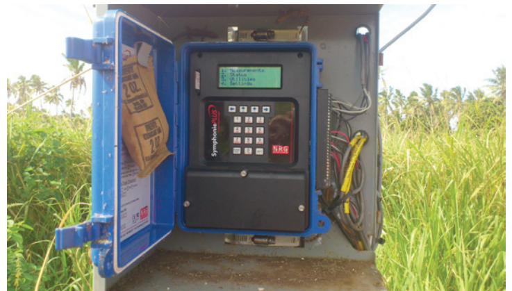
Data logger for recording wind measurements at the bottom of the Lapaha wind monitoring mast, photo: Kevin Palmer-Wilson, GIZ
