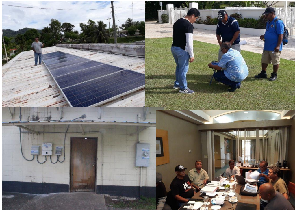
Photos: Left top and bottom: Kosrae 3.25 kW solar with inverter and net meter installation at KUA administration building Right top and bottom - Participants at the Solar PV grid connected training in Guam
