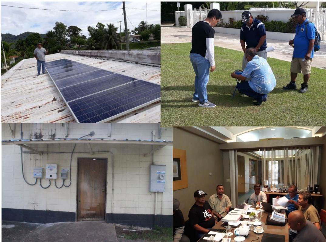
Photos: Left top and bottom: Kosrae 3.25 kW installation with inverter and net meter at KUA administration building Right top and bottom - Participants at the Solar PV grid connected training in Guam
