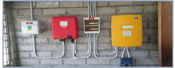
Figure 5. solar inverters and controller at the JSS
