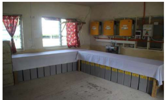
Figure 11. Solar energy systems inverters and battery
