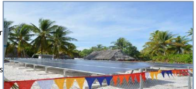
Figure 1. ASMC 20 kW solar panels ground mounted installation, Abemama Island
