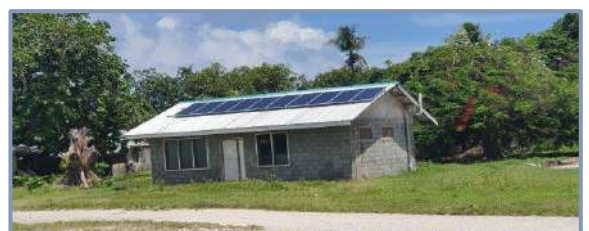
Figure 4. 5kW solar installation at Police Post, Teraina
