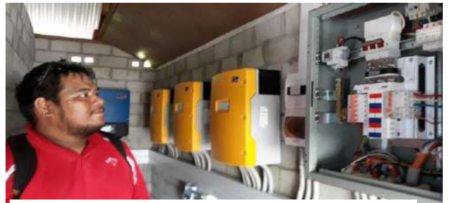
Figure 2. Solar inverters and controllers, Teraina JSS
