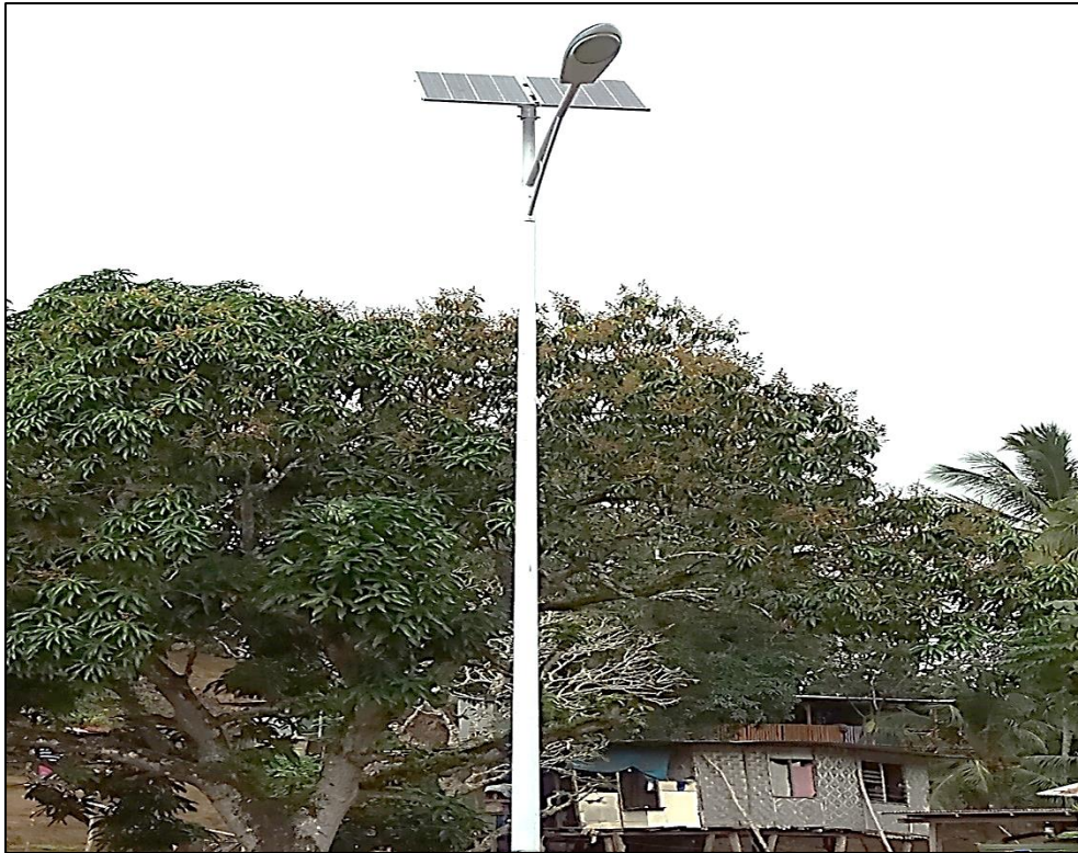
Figure 22: Solar panel need to be re-orientated to face the north
