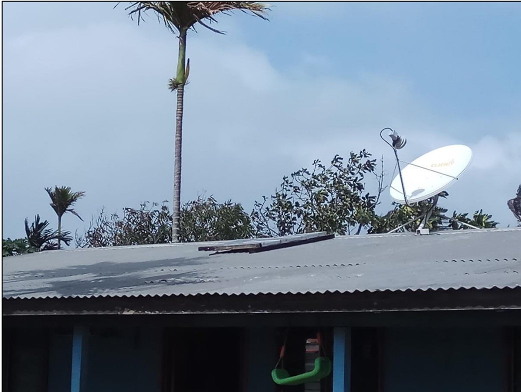
Figure 20: Solar panel on roof to power the TV reception disk in Keapara
